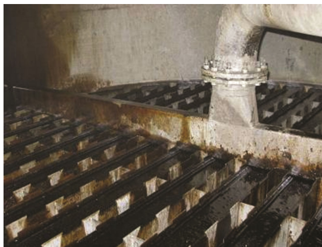
Fig. 1 — Detail of the built-in structure of the hydrogen-sulphide scrubber
