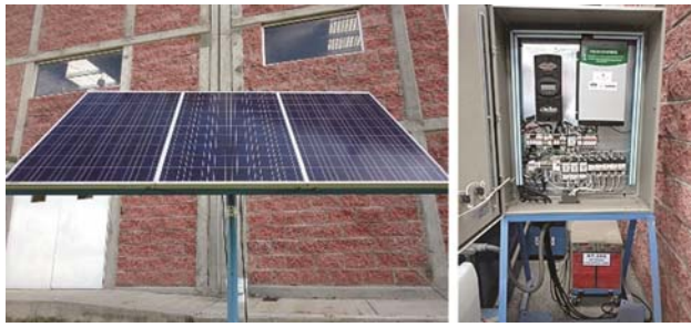
Fig. 5 — Photovoltaic panel, control panel, and battery bank
